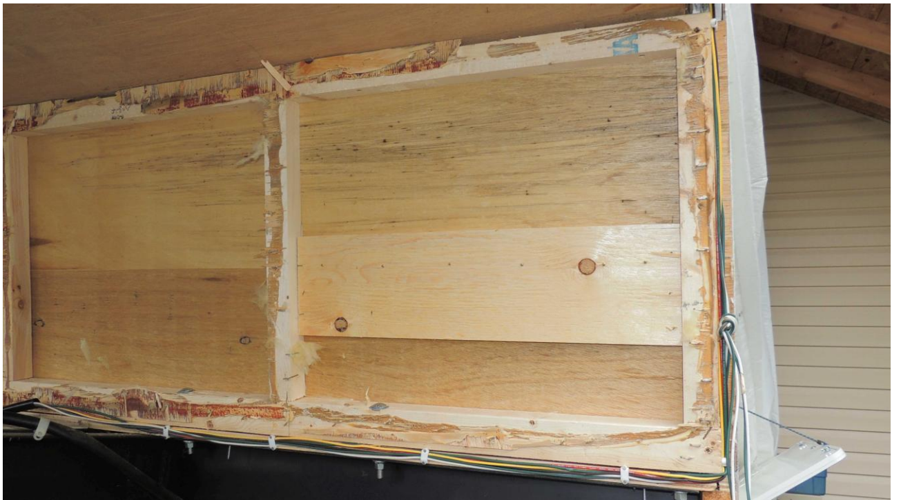
Driver's side kneewall, after removing the front plywood, no damage at all.
