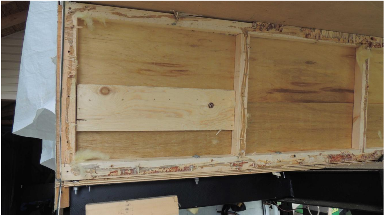
Passenger's side kneewall, after removing the front plywood, no damage at all.
