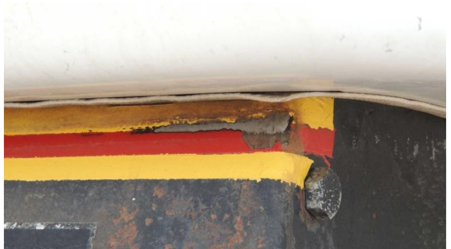
Before the repair: one inch deflection.
